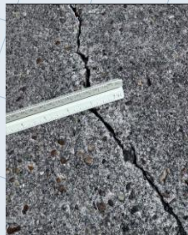
Detail of 1/4 inch crack on the deck surface
