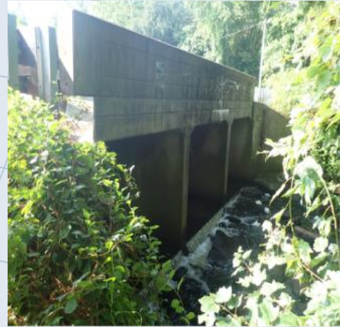
Efflorescence, showing as white leaching down the side of exterior wall, is a sign of minor chemical reaction in the concrete.
