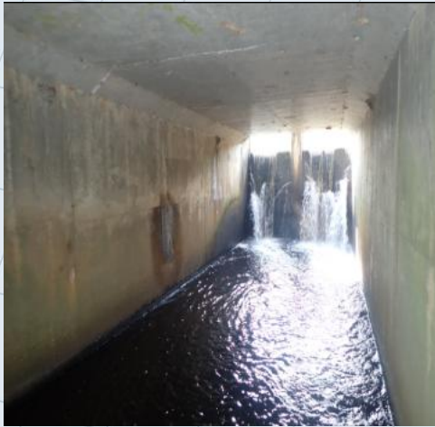
Rust staining on interior walls of the culvert is a sign that water and other fluids are getting into the structure.
